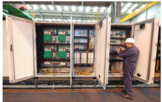
ABOVE: The adoption of common drives, PLCs, HMIs and control gear provides spares compatibility, reduces costs and enables operator training to be standardised. In addition, it has enabled Transicon to incorporate numerous additional safety and diagnostics capabilities within the upgraded installation.
